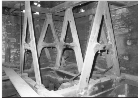
Temple Church bell-chamber to-day. Cast-iron A frame by John Taylor & Co, 1887. The chiming hammers were added in 1935 and the bells removed in 1941
